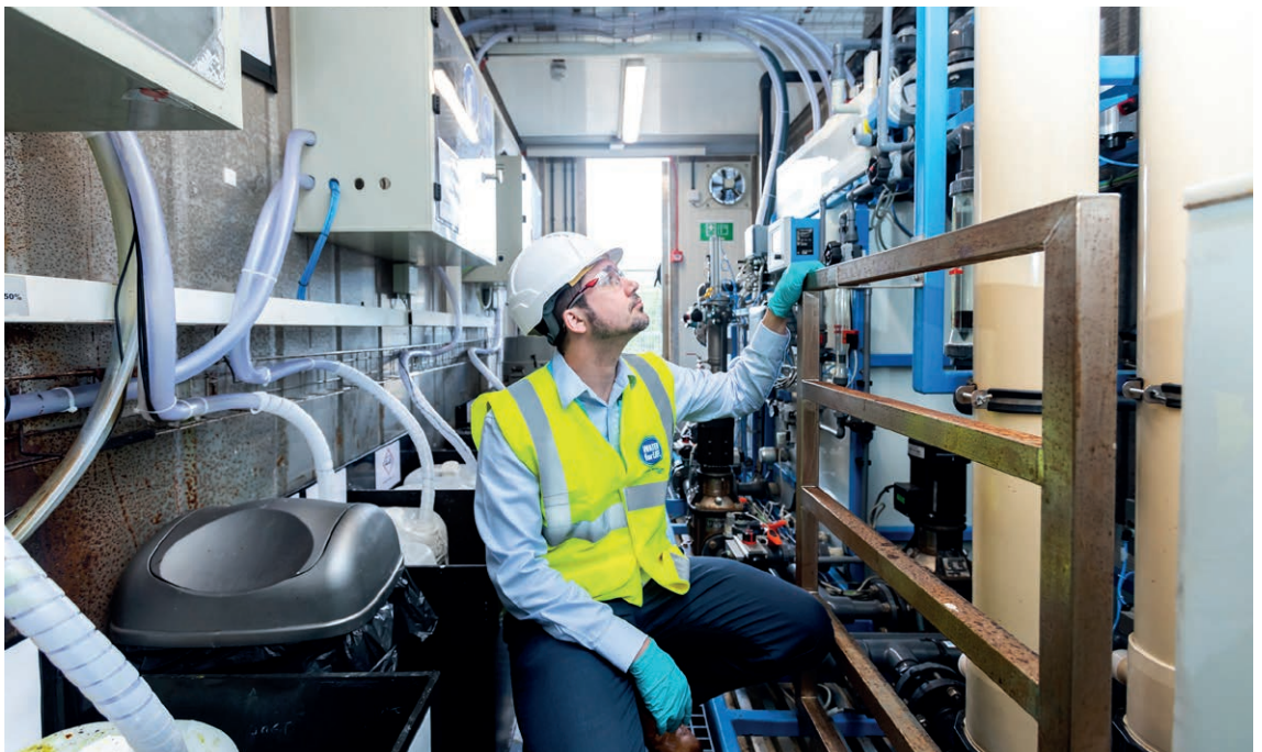
Peel Common Wastewater Recycling pilot.
